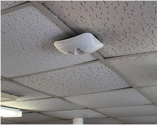
Picture 1 - WAP in Room 138
