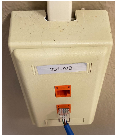
Picture 6 - Ethernet plugs only present Rooms 231 & 222
