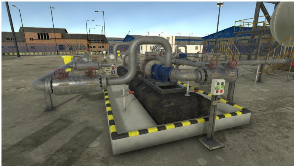
Figure 6 – Duty and Standby water pump
